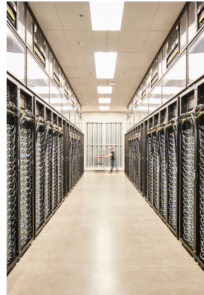
Apple's Reno data centre, opened in 2012, takes advantage of the mild climate by cooling its servers with outside air whenever possible.
